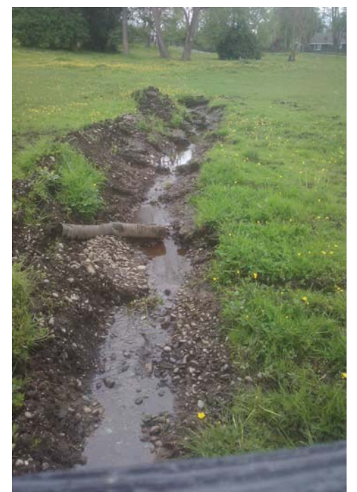
Improperly trying to solve drainage issues may garner you a fine, especially if you impact nearby waterways or county ditches.
