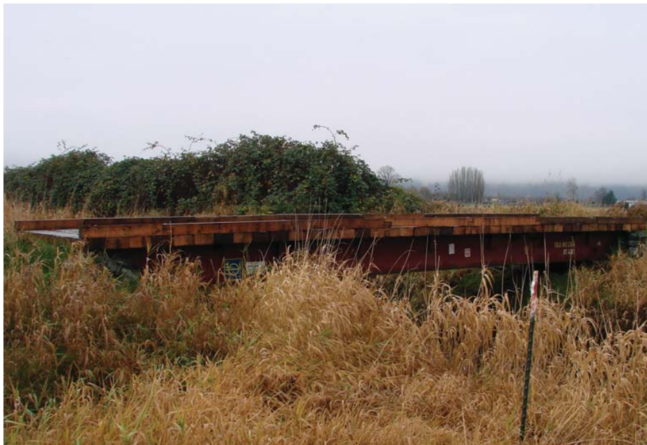
The new 'recycled' bridge keeps water from backing up and improves fish passage in Swan's Trail Slough.
