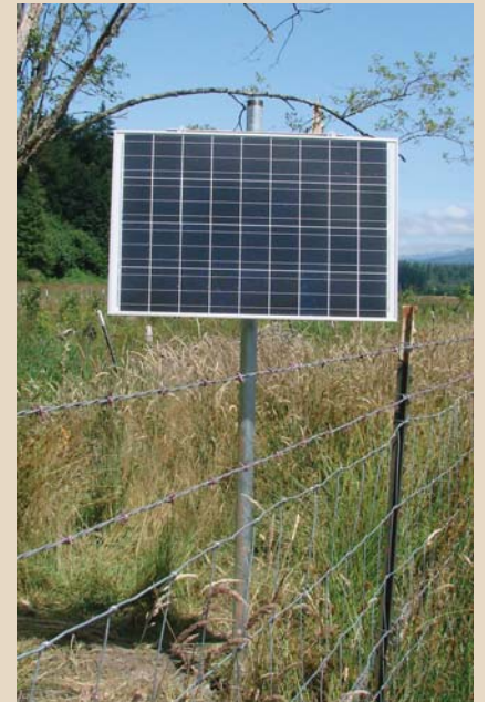
The collection panel is safely tucked behind a fence.
