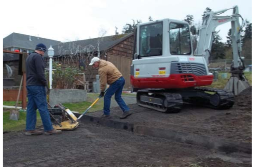
Chris Crouch of EarthFirst Construction and District Engineer Kelly Cahill use a plate compactor to compact crushed gravel just below the rubber diverter.
