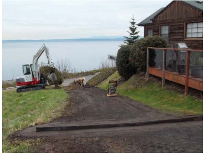
With one deflector in (foreground), another is being installed below. Surface water is diverted to the pasture on the left. With Puget Sound directly below this neighborhood, it's crucial to control erosion.
